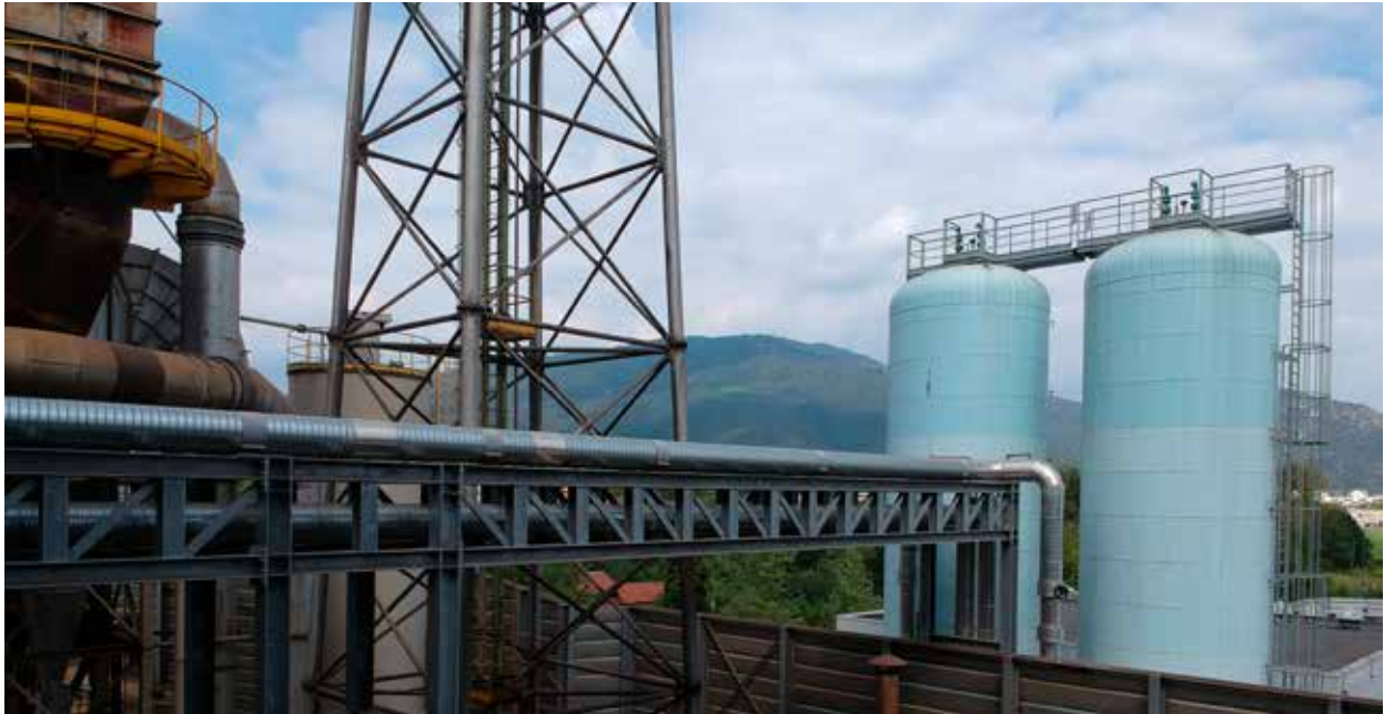
Alfa Acciai: array of pipes supplying the heat recovery plant from the steel mill and storage tanks
